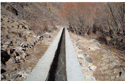
Photo: Improved irrigation canal in Dome-Jangal, Saighan. 120 families benefit from this canal.
