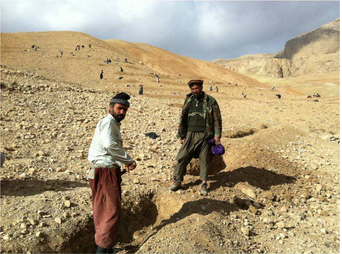
Photo: People from Roy-e Sang village constructing contour trenches in Sourakhak watershed, Kahmard, with a cash for work approach.
