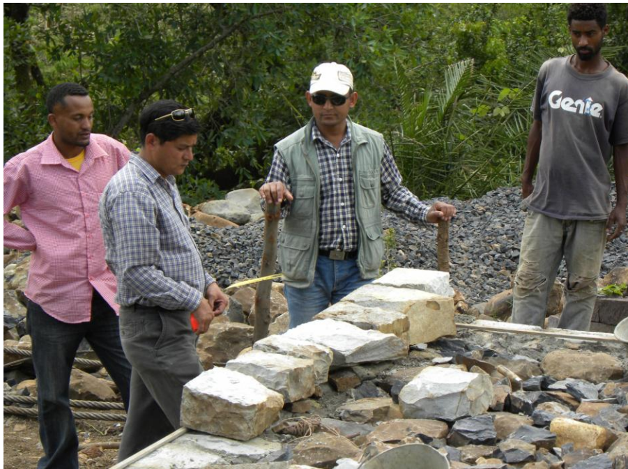
Backstopping by Nepali trail bridge technical officer about masonry structure, March 2010, Ethiopia
